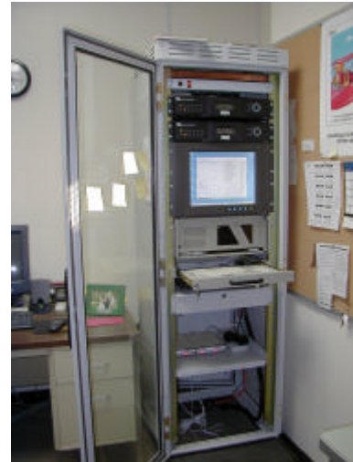
MASTER RADIO STATION EQUIPMENT RACK
