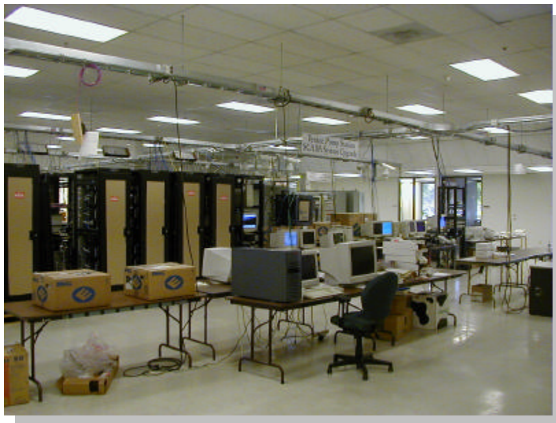
FACTORY TEST AT TRANSDYN CONTROLS
